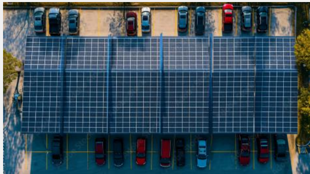
Solar carports (car shelter + solar power plant)
