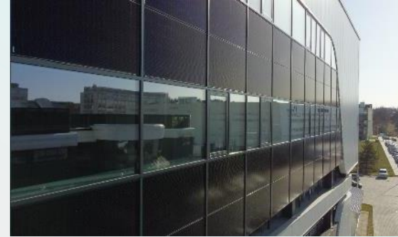
Building facade-integrated solar panels
