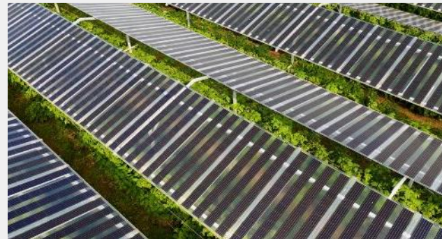
Agro PV integrated solar greenhouse
